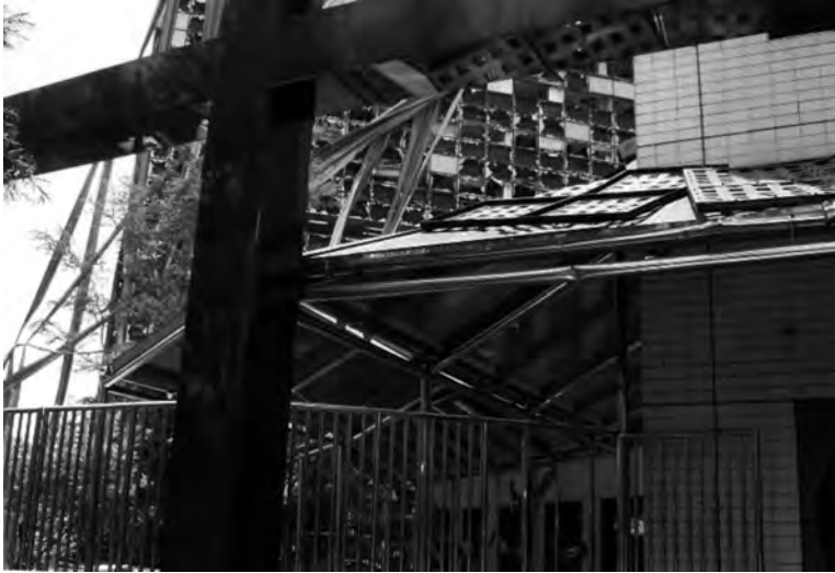
Figure 35.5 Damage to the Australian embassy and surrounding buildings (photographer courtesy of the author)
